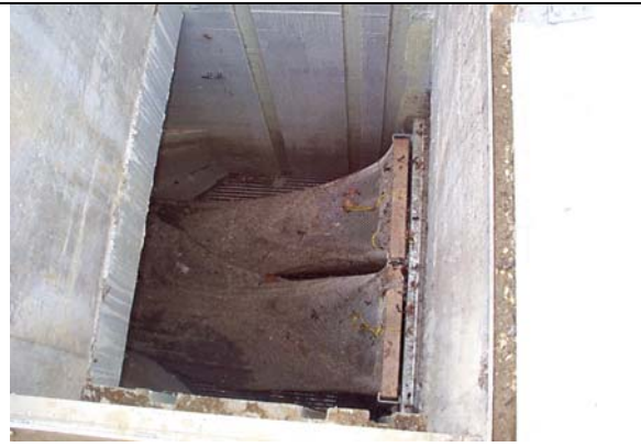
Figure 4: Photo of Nets installed in T-4 CSO Outfall
