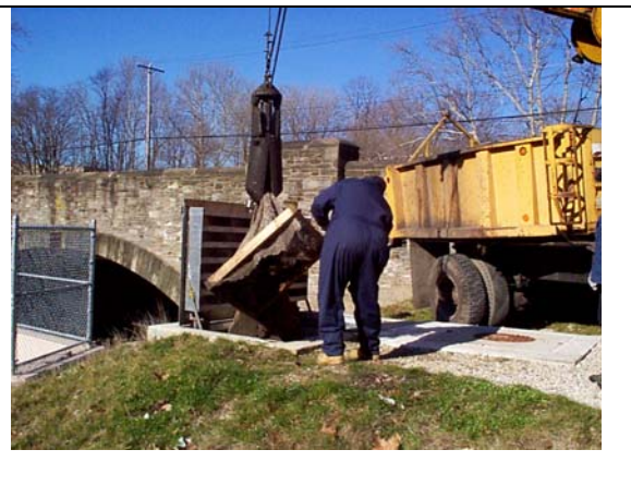
Figure 6: Maintenance of floatables nets at T-04
