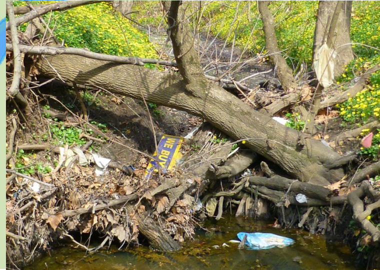
B. Outfall channel by woody debris jam
